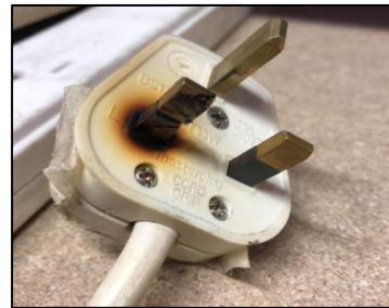
Plug top showing signs of overheating
