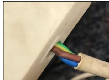
Exposed bare wires
