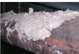
Fig 3: Amosite pipe lagging in very poor condition.
