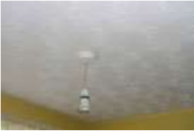
Fig 3: Asbestos textured coating (artex) on ceiling.
