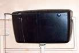
Fig 4: Toilet cistern containing reinforced asbestos materials.
