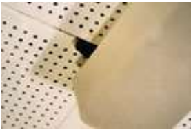
Fig 4: Damaged perforated ceiling tile
