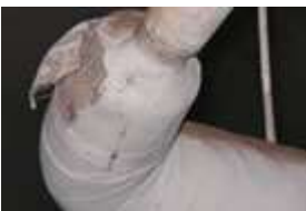
Fig 1: Damaged asbestos pipe lagging.
