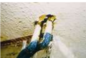
Fig 2: Damaged asbestos coating around pipework.
