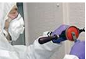
Fig 1: Asbestos textured coating on wall.
