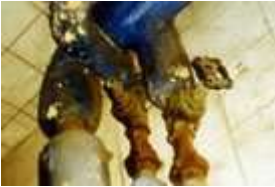
Fig 4: Asbestos lagging on hot water pipes.
