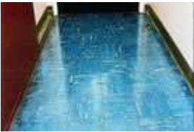
Fig 3: Asbestos containing vinyl floor tiles.
