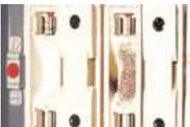
Fig 2: Asbestos flash guards in fuse box.
