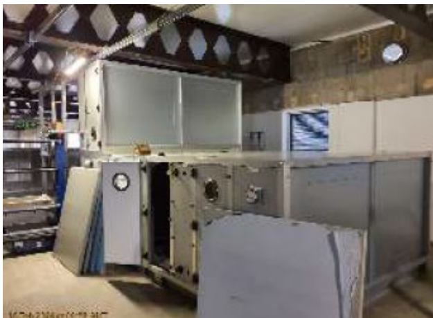
Refurb – First Floor Plant Room - ATC / CAU air handling unit delivered and being installed
